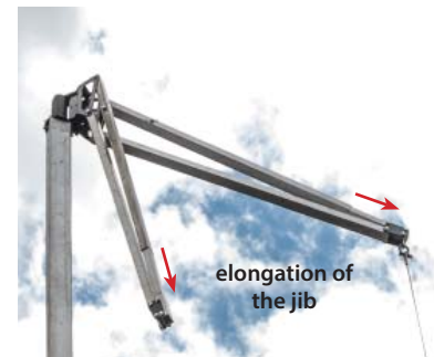
Figure 21a Overload Indication.
